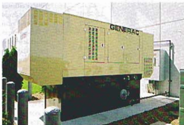
A proper UPS system design will incorporate generators into the mix as support and backup.
